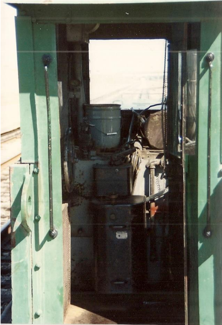
A look inside the operator's cab.
