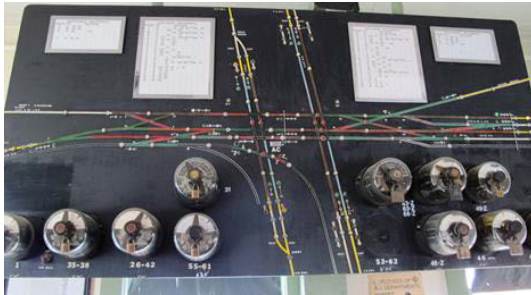
Photo 6. A close-up view of the restored model board. The tower was donated to the Marion Union Station Association in 1995 by Conrail, and was moved from its original site across the depot to the depot grounds. The restored model board shows the pre-Conrail track alignment, with the Erie and New York Central lines going from left to right, and the Pennsylvania and Chesapeake and Ohio main lines going top to bottom (right and left, respectively). The round glass devices are mechanical timers which are part of the intricate system used to protect trains moving through the interlocking plant.
