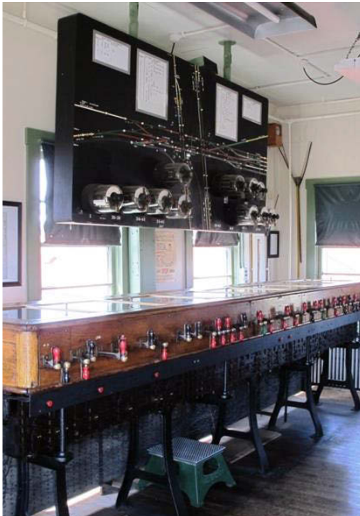
Photo 5. The Taylor interlocking machine in AC Tower. The top of the cabinet is glass, allowing viewers to look into the cabinets and see the electrical and mechanical connections. Underneath the front face of the cabinet (the black panel below the red buttons) are the mechanical interlocking tabs for the machine.
